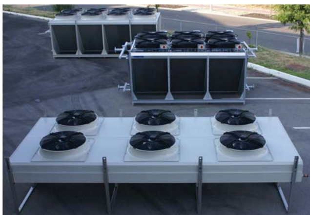
Condensadores ACPD e VACD ACPD and VACD condensers
